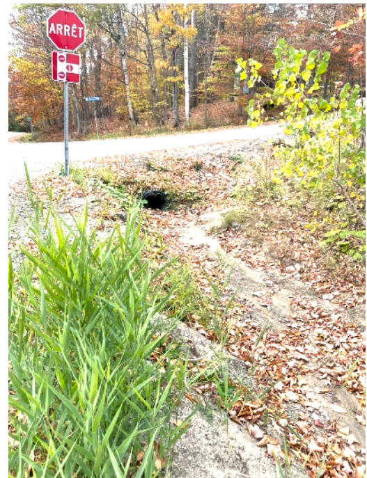
An example of an unstable ditch (corner of Forest Hill & Lakeshore), showing accumulation of sediment and establishment of an invasive plant species (phragmites)
